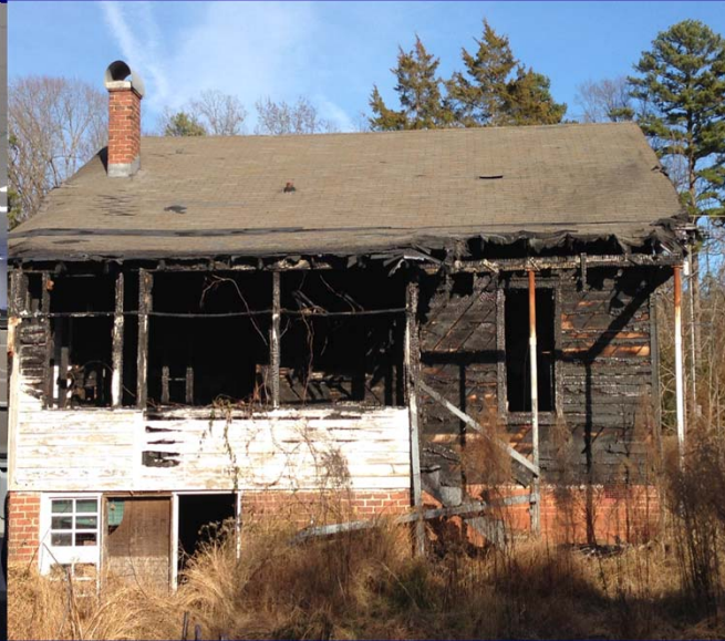
Fire damaged house allocated to Department of Public Safety (not listed as part of the state inventory)
